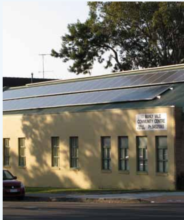
Top: Power-Mate Lite. Source: Warringah Council. Above: Solar Panels at Manly Vale Community Centre. Source: Warringah Council
