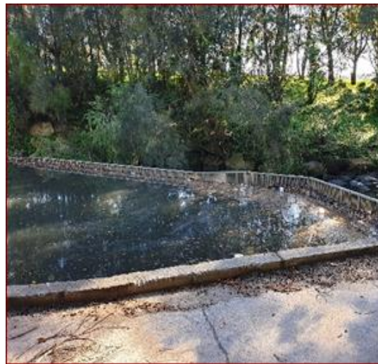
Photo 7: GPT trash rack (looking downstream)
