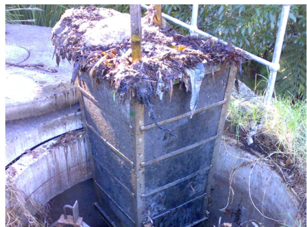
Cleaning of Clontarf gross pollutant trap. Source: Manly Council.
