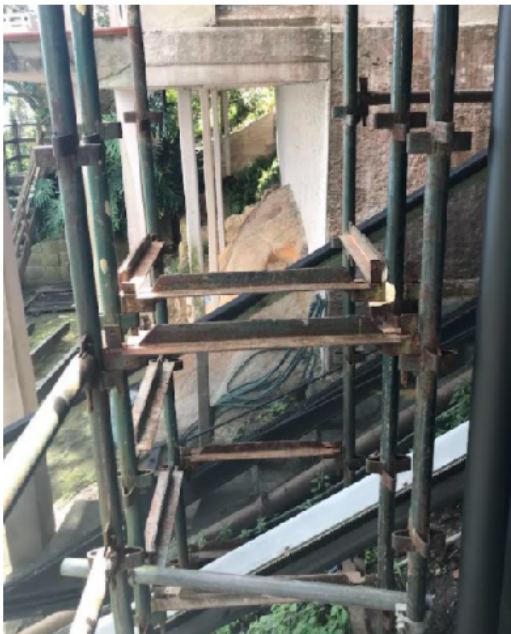
Photo 3: Relationship of the inclinator platform servicing Level 1 of the Studio to the southern adjoining property.
