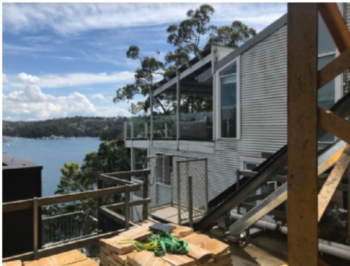
Photo 2: Relationship of the upper additional and repositioned inclinator landings to the southern adjoining property.
