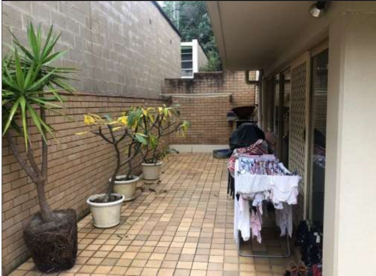
Image: Area of additions across part of the ground level side terrace (Unit 1) and the adjacent neighbouring solid wall.
