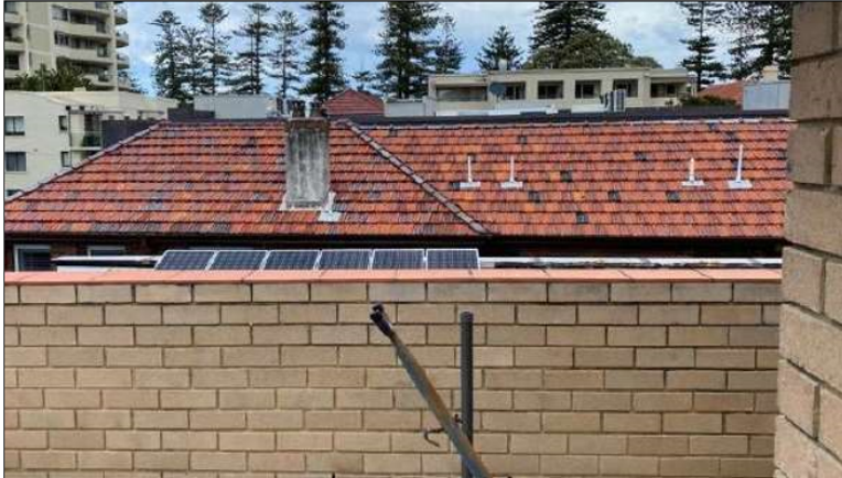
Image: Southern side of terrace at location of additions to roof area. Note solar panel on adjacent roof.
