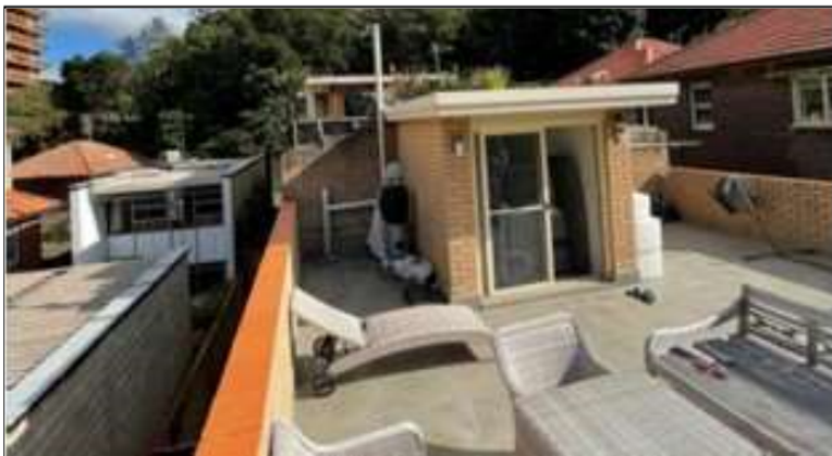
Image: Area to be enclosed for roof additions (rumpus and bathroom) for Unit 5 terrace on either side of stair access.
