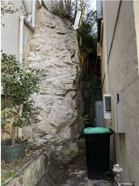
Figure 12 - character of existing rock excavation to accommodate the existing dwelling - eastern side
