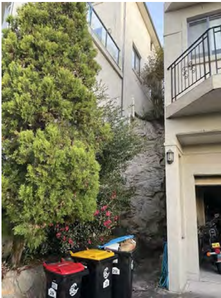
Figure 11 – character of existing rock excavation to accommodate the existing dwelling - eastern side
